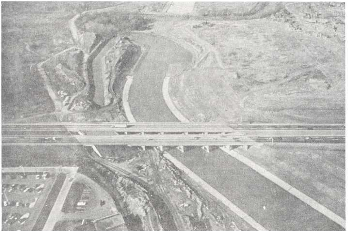
Looking approximately northwest toward the Edsel Ford Bridge (I-94) in Dearborn. Shown here is the completion of Section A and the beginning construction of Section B. Courtesy: Dearborn Times-Herald .
