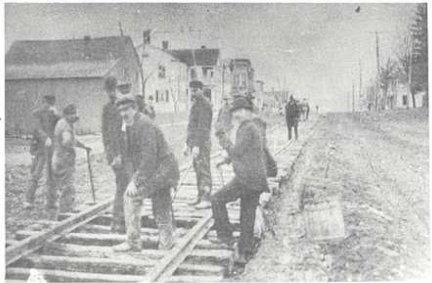
Laying tracks for the Detroit, Ypsilanti, Ann Arbor and Jackson Railway just east of Center (Monroe) Street on Michigan Avenue in December of 1897. [Museum Collection]
